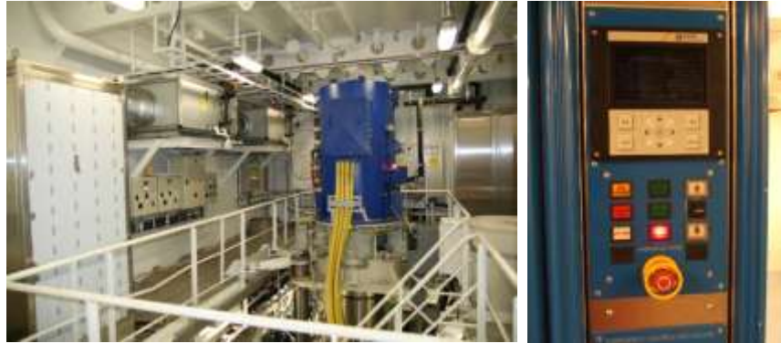
Electric Propulsion Motor
