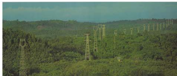
230KV TRANSMISSION LINE (THAUK YAE KHAT - TAUNGOO)
