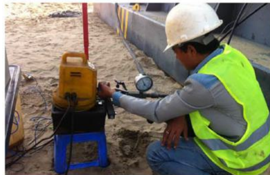
Operating Electric Pump
