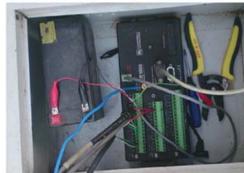
Data Logger Panel
