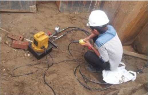
Operating Electric Pump
