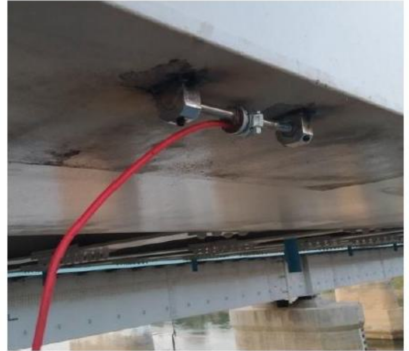
VWSG Installation Photos
