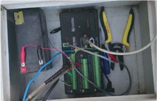
Data Logger Panel
