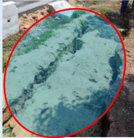
Liquefaction near 145 Milestone
