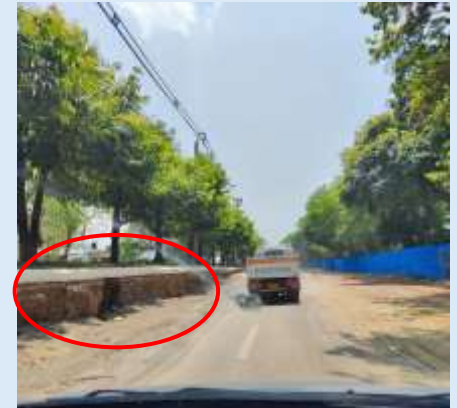
Road collapse Sagaing-Mdy Road
