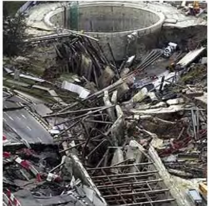
(b). After collapse
