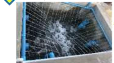
Primary Sedimentation Tank
