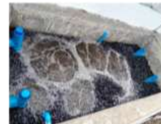
Moving Bed Bio-reactor Tank (BOD Removal)
