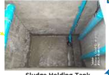
Sludge Holding Tank
