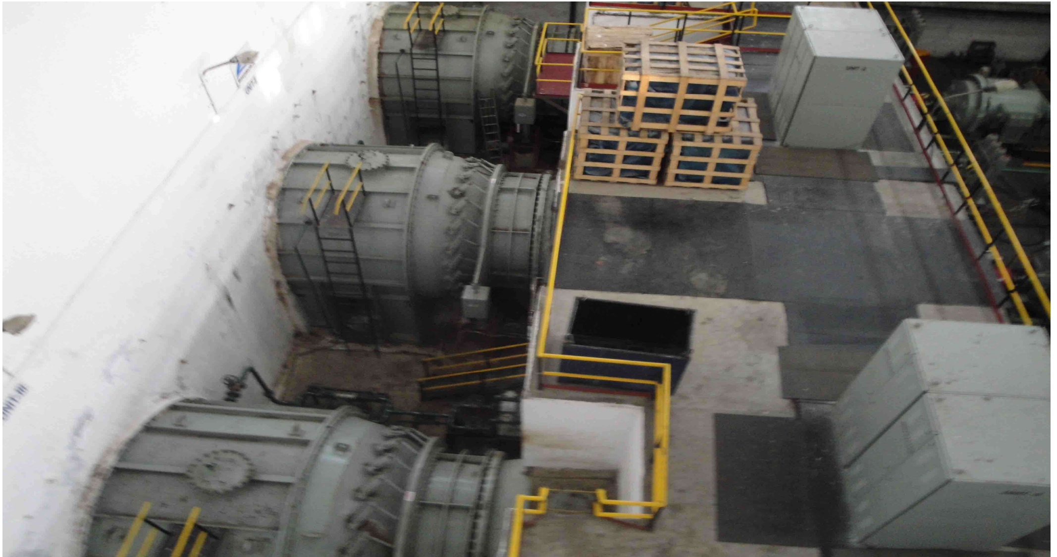
Fig. 41: Turbines and Control Panels View
