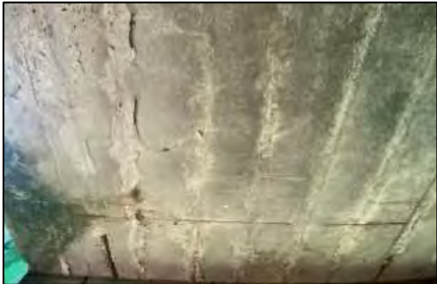
Prone to Spalling
