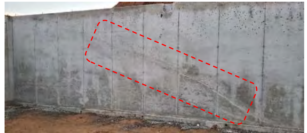
Cold Joint in Wall
