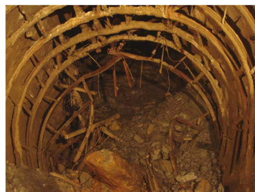
Figure 25 Collapse of wrong excavation technique.
