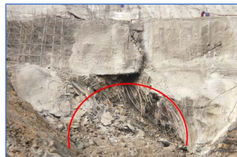
Figure 24 Improper support system.
